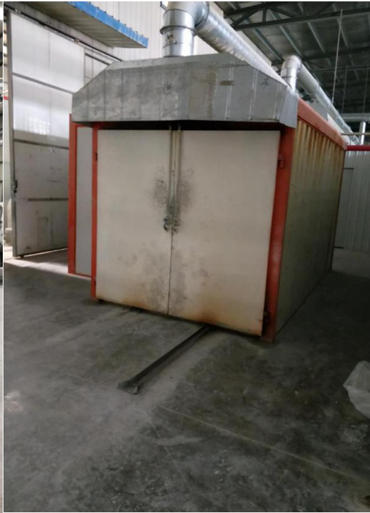
图为整改后中涂烘干室废气收集罩
